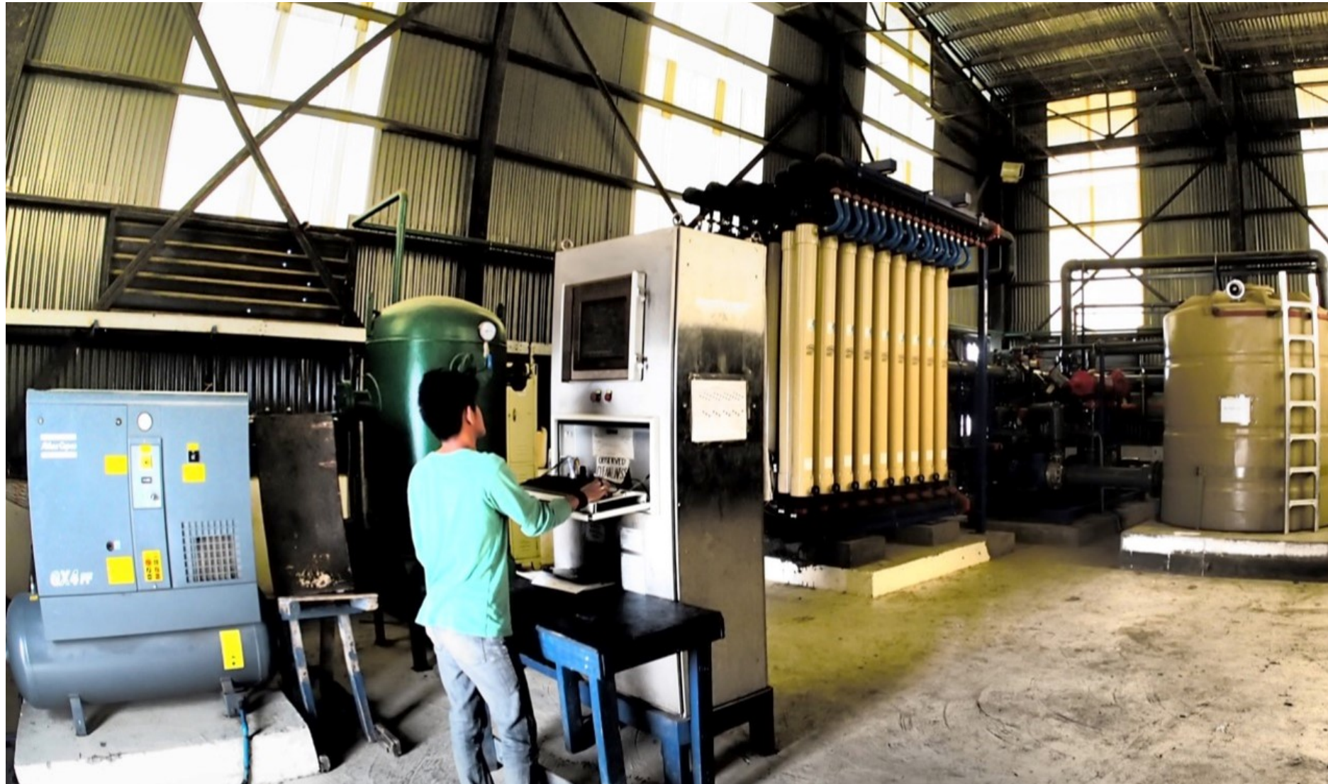
Water filtration facility – Semirara Island
